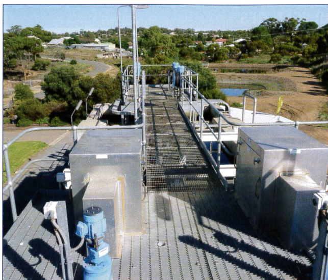
Optimised coagulation with minimised polymer dosing can reduce NDMA at some plants. See page 76.
