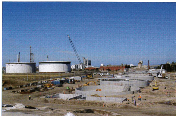
Northern Water's $94 million Class A recycled water plant under construction at Geelong in Victoria. See page 22.
